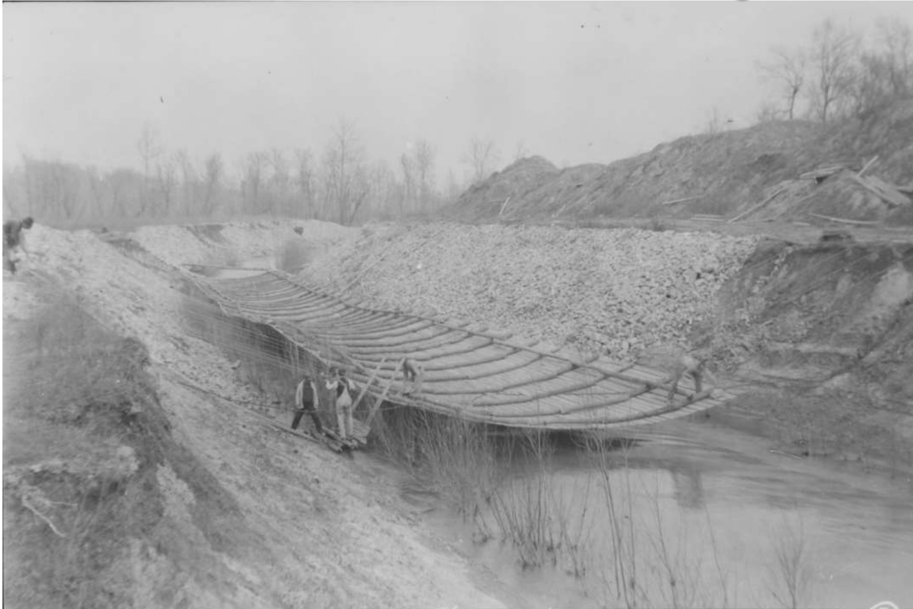
Board Mattress Sta. 640 CR. Div. Ch. Placing stone at up stream end. (2)
