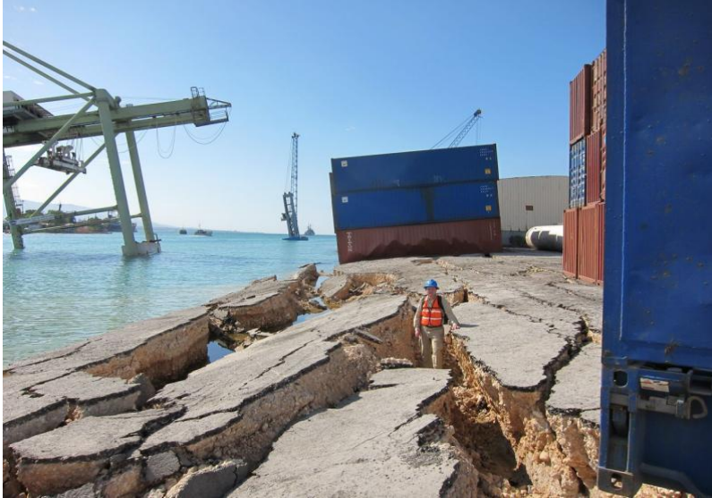
USGS/EERI Haiti EQ Damage report
