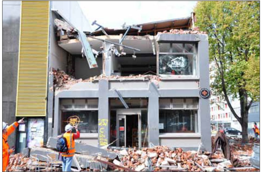
Figure 15. The EERI Team studies the performance of this heavily damaged, retrofitted URM building that pounded against the building on the left and partially collapsed (photo: Turner).
