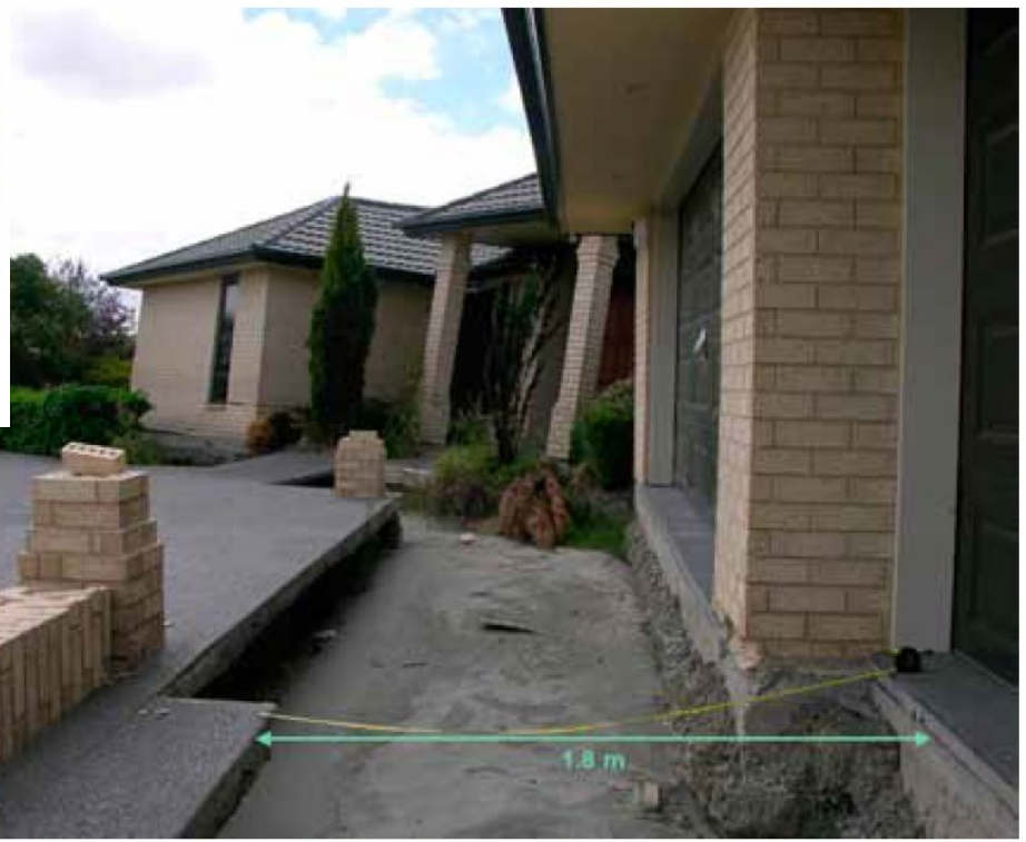
Figure 21. A house in Kaiapoi moved on its foundation in both the September and February earthquakes a total of 1.8m (photo: Lai).
