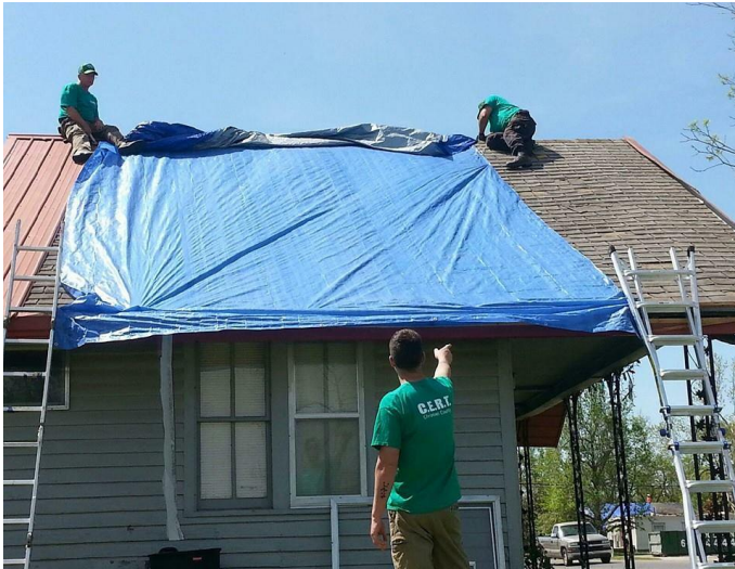
MOCERT1 team members work on a roof damaged by a tornado in Baxter Springs, Kan.
