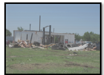
Tornado damaged gas station in Eureka, Kansas Photo Credit: Steve Samuelson, Kansas State NFIP Coordinator
